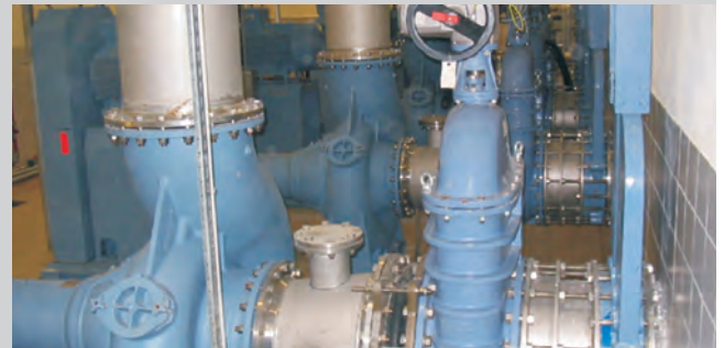
Pumping station at the stormwater overflow basin in Dresden-Kaditz
